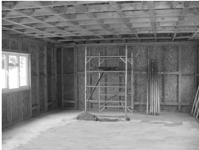
Stage Six: internal timbers and foundation raft. NB all sections are bolted to each other and down to the foundation raft
